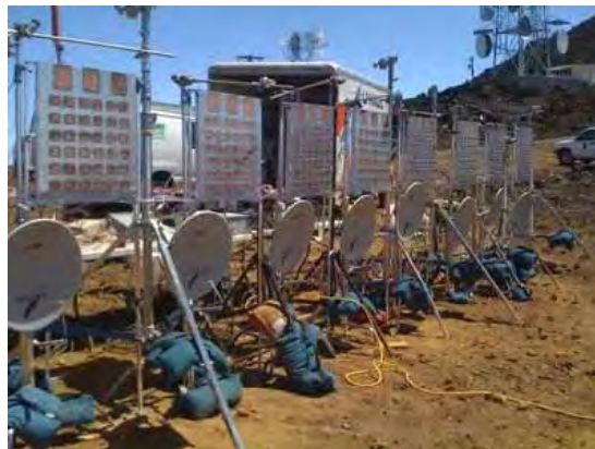
An array of microwave power transmitters set up on Haleakala for the power beaming demonstration. (courtesy of National Space Society)
